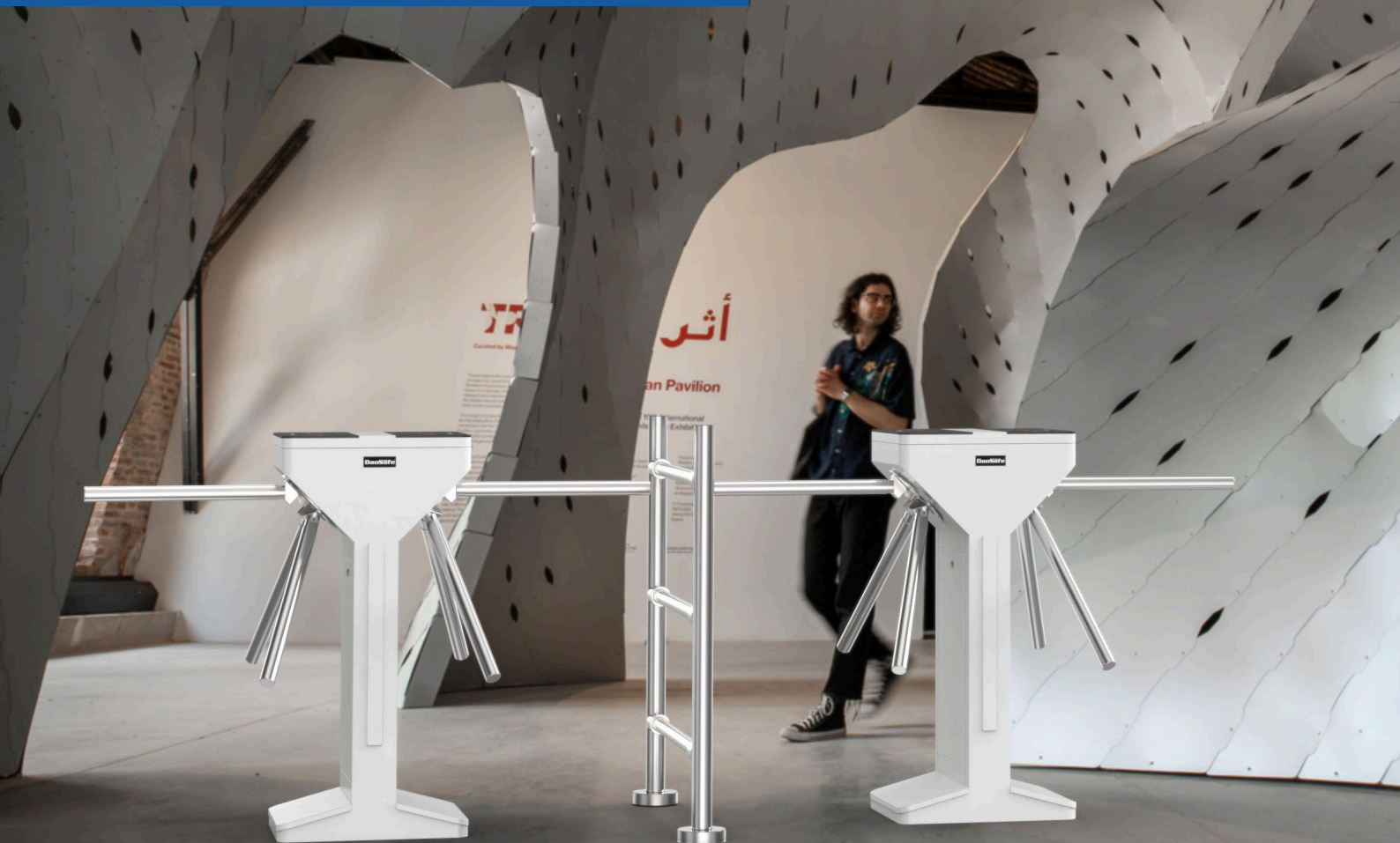
4 lanes DS-Q50 customized color installed at entrance
