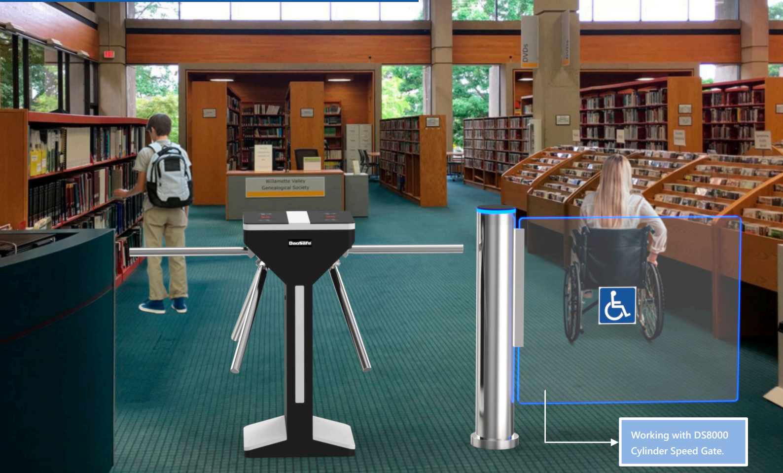
DS-Q50S and DS8000 disabled lane installed at library
